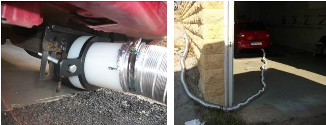
Fig. 3.11. Exhaust extraction system
