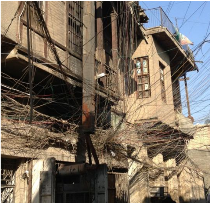
Figure 57: A traditional building with an electric generator serving the neighborhood. The generator occupies the ground floor of the building.
