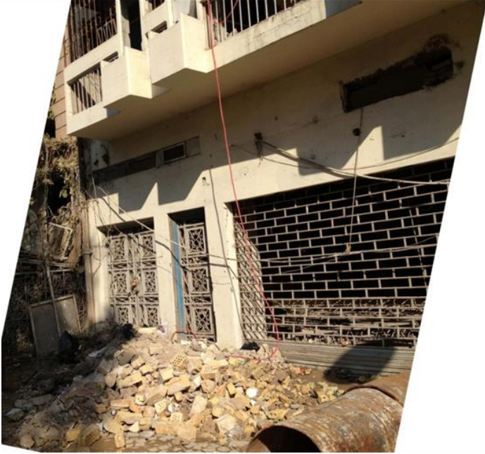
Figure 25: Abandoned ground-floor shops of one of the buildings with construction waste on the sidewalk in front of it.
