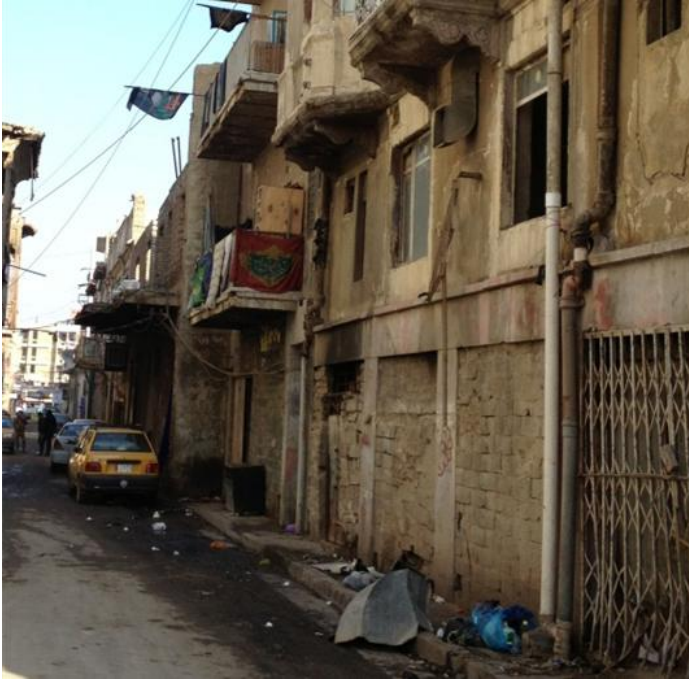
Figure 58: Ground-floor shops closed-off with bricks. Note the dilapidated condition of the old traditional buildings.
