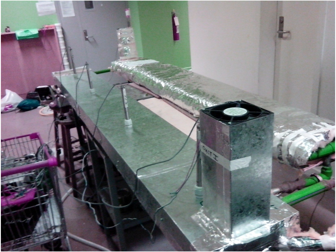
Figure 16: Photo showing the sensors placed across the dehumidifier
