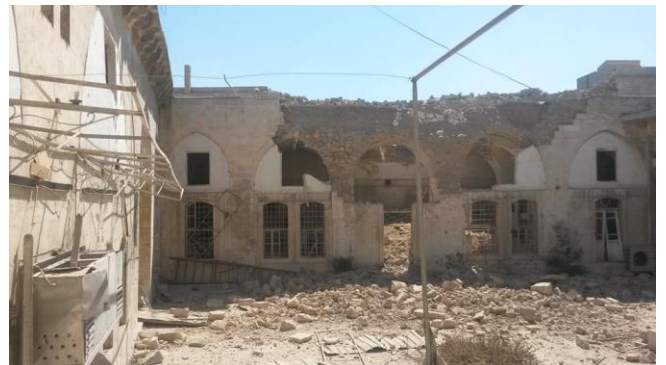
Figure 117. Image showing the destruction of the internal facade Source: Retrieved 2014 from http://joh7fais.wordpress.com/
