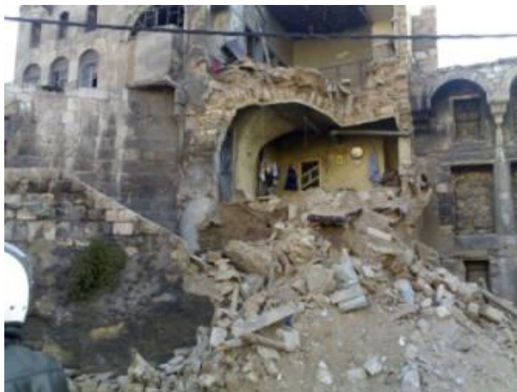
Figure 69. Image showing the destruction of the façade in Qadi Askar boulevard area
