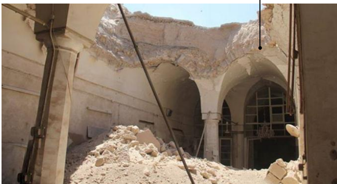
Figure 115. Image showing an inside view of the destroyed ceiling of the mosque Source: Retrieved 2014 from http://ioh7fais.wordpress.com/
