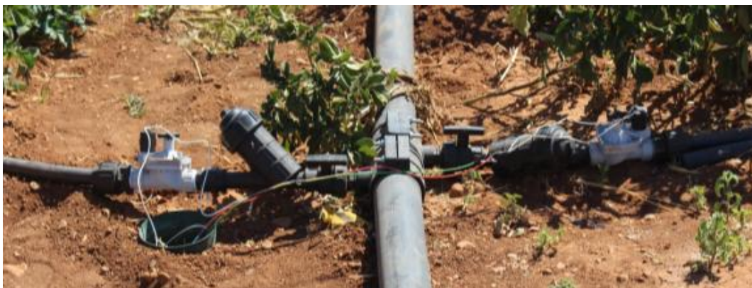
Fig. 14. Solenoid valves, filter connected to the controller
