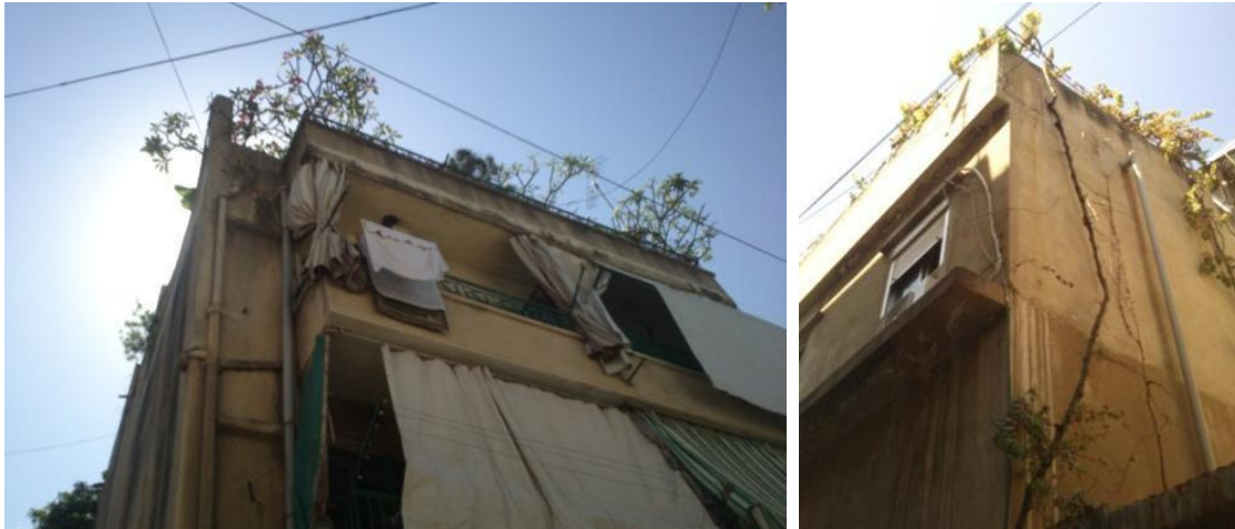
Figure 77: Nabaa's green roofs. Many residents grow on their roofs grape vines or other ornamental trees
