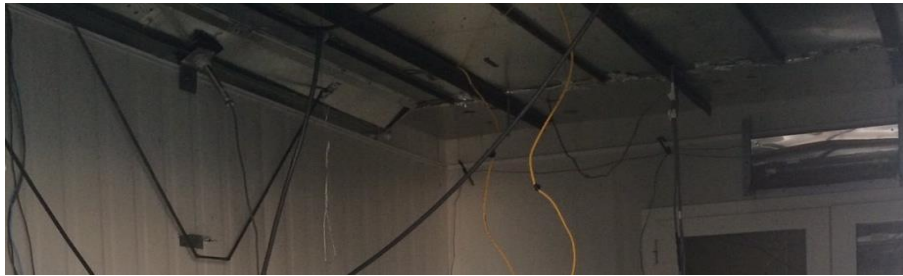
Figure 6: Exhaust Grill Connected to the Ceiling of the Experimental Setup
