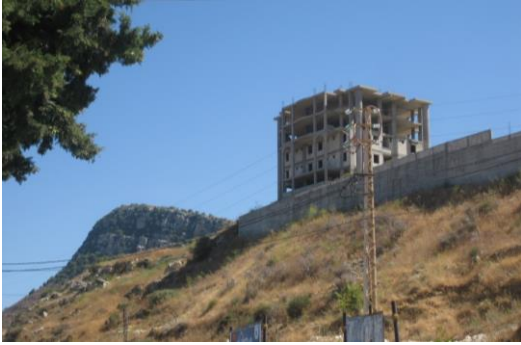
Figure 4. New building under construction in Jezzine town. This photo illustrates how the new developments are out of scale and does not relate to the surroundings. Photo Taken by Neaimeh, R.
