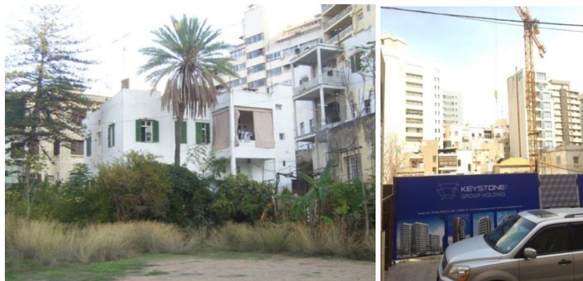
Figure 62: A construction site replaces an old building on Rawda Street (Gebara, H., 2016)
