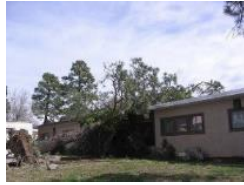
Wind, damage, reported gust
