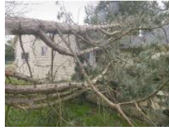
Hurt, tornado, winds, damage
