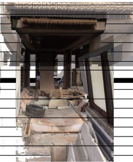
machine : gang saw health concern : dust / noise pollution
