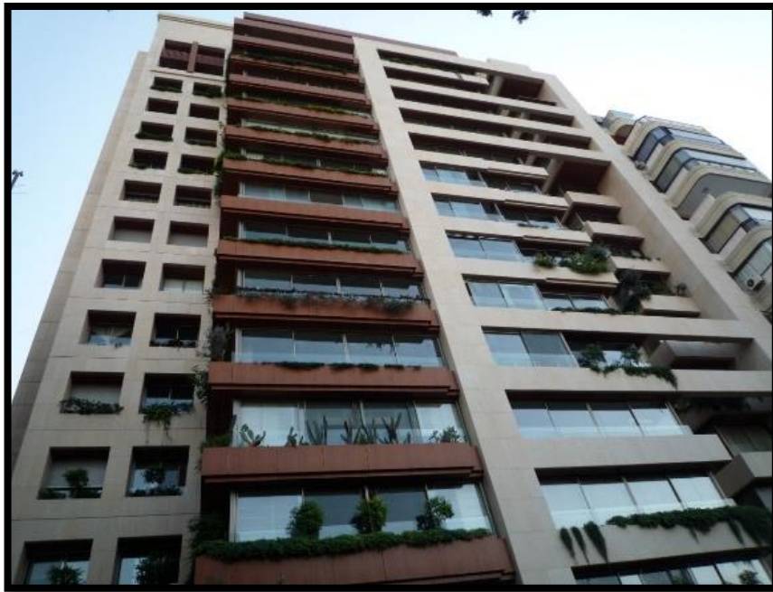
Figure 42 Existing building with dangling vegetation from wall planters
