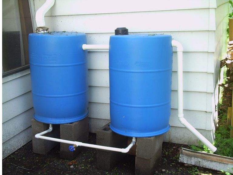
Figure 15 Rain barrels for rainwater harvesting (Source: www.offgridquest.com )
