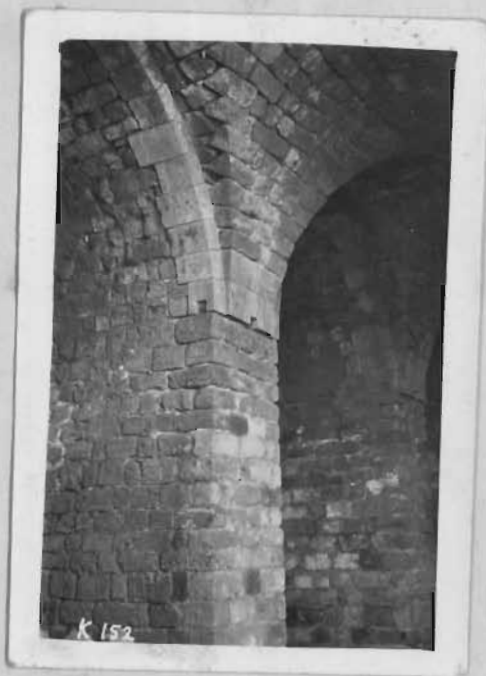
Photo N° 27 showing an Arab goined vault construction of XIV century, Tower of Lions tripoli, note the use of Crusaders solution for the goined arch corner and timidity in cross vaulting expressed by the use of stereotommed arc.
