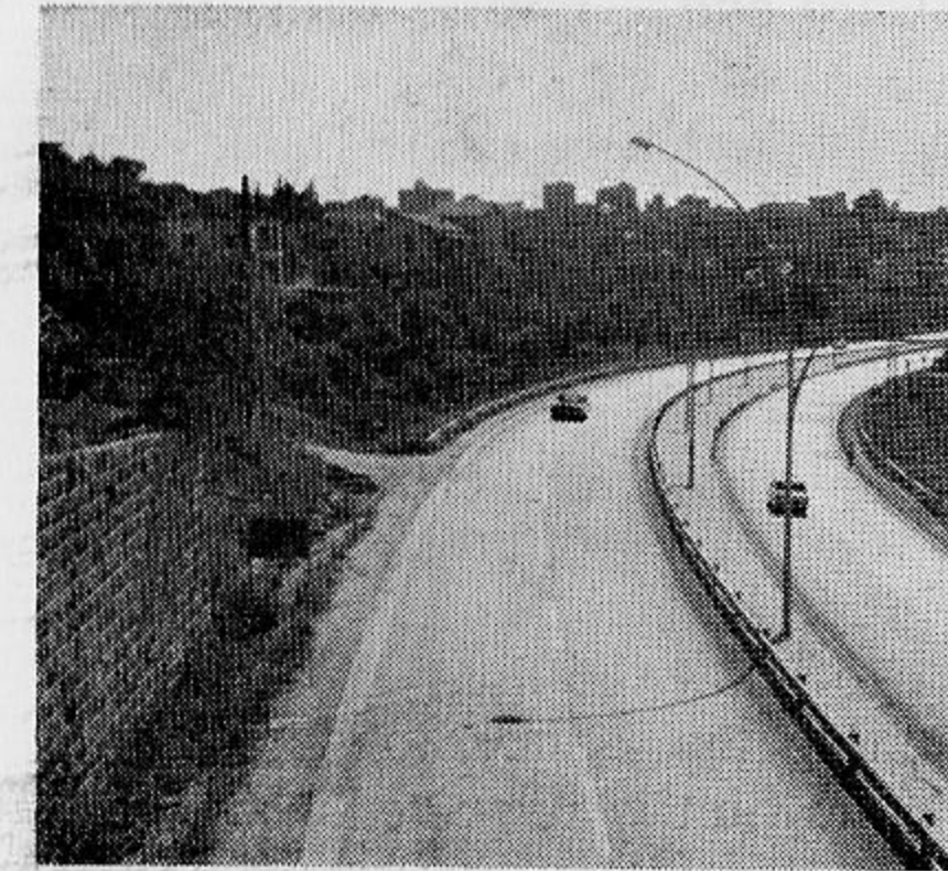
Figure No. 16 Split level median with guardrail - type C - Upper roadway on horizontal curve Location under study
