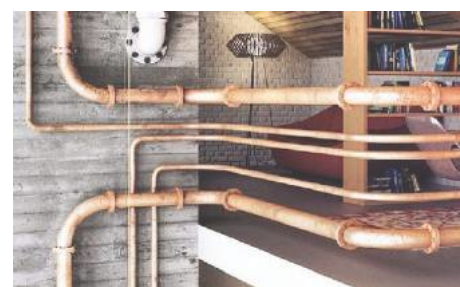
Main Pipeline | Lighting and Handrail
