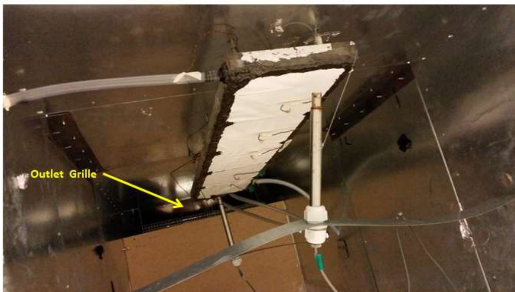
Figure 14: Dehumidifier installed inside the chamber
