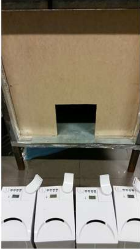
Figure 15: Air supply grille and humidifiers
