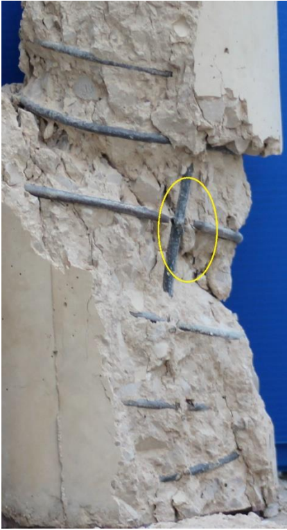
Figure 40. Spiral hoop failure
