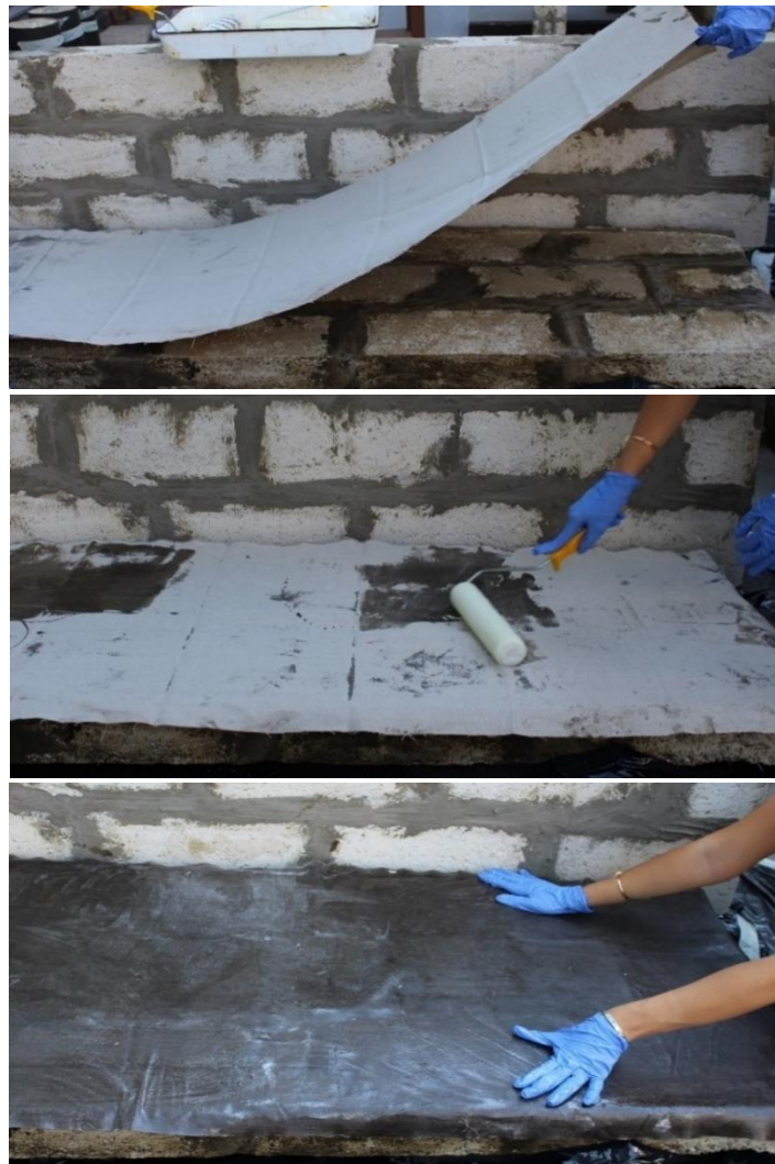
Figure 3.23 Installation of Hemp Fabric to Masonry Wall (Series H1, H2, and H3).
