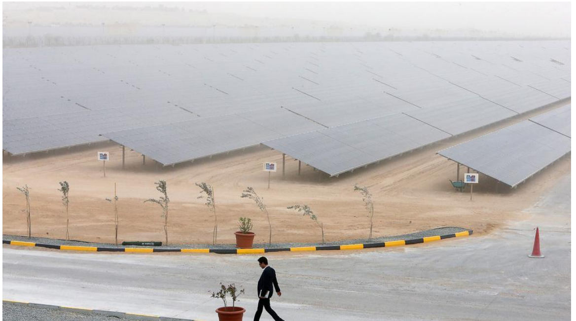
Figure 14. Mohammed bin Rashid Al Maktoum solar park
