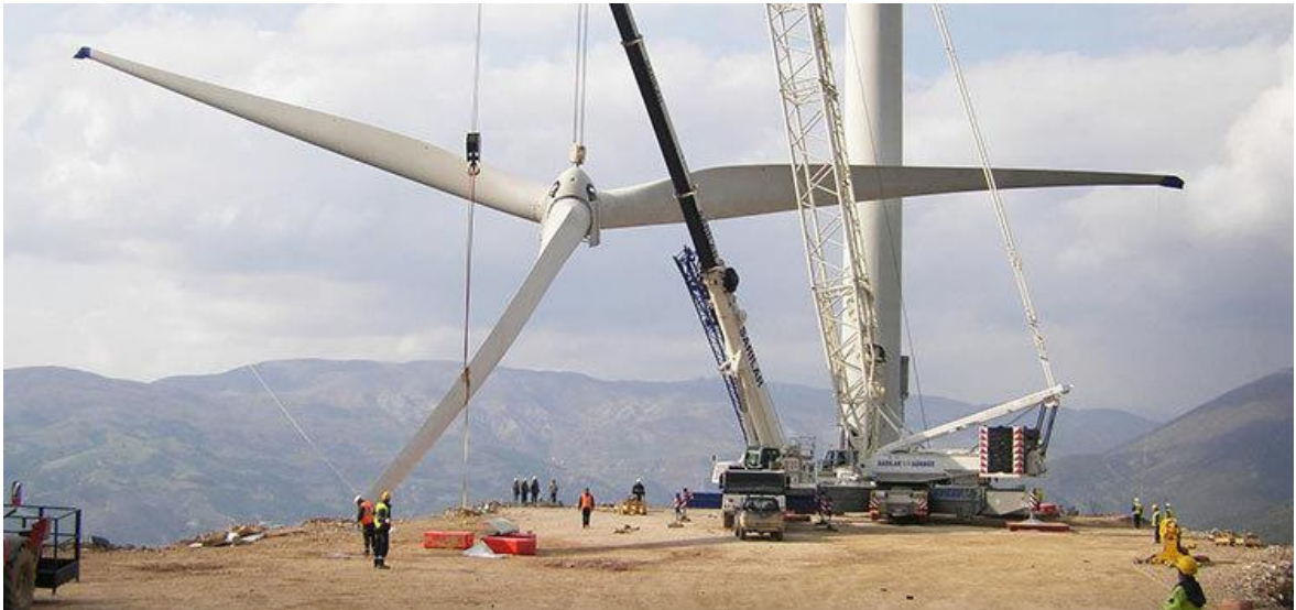
Figure 13. Al Rajef wind power plant
