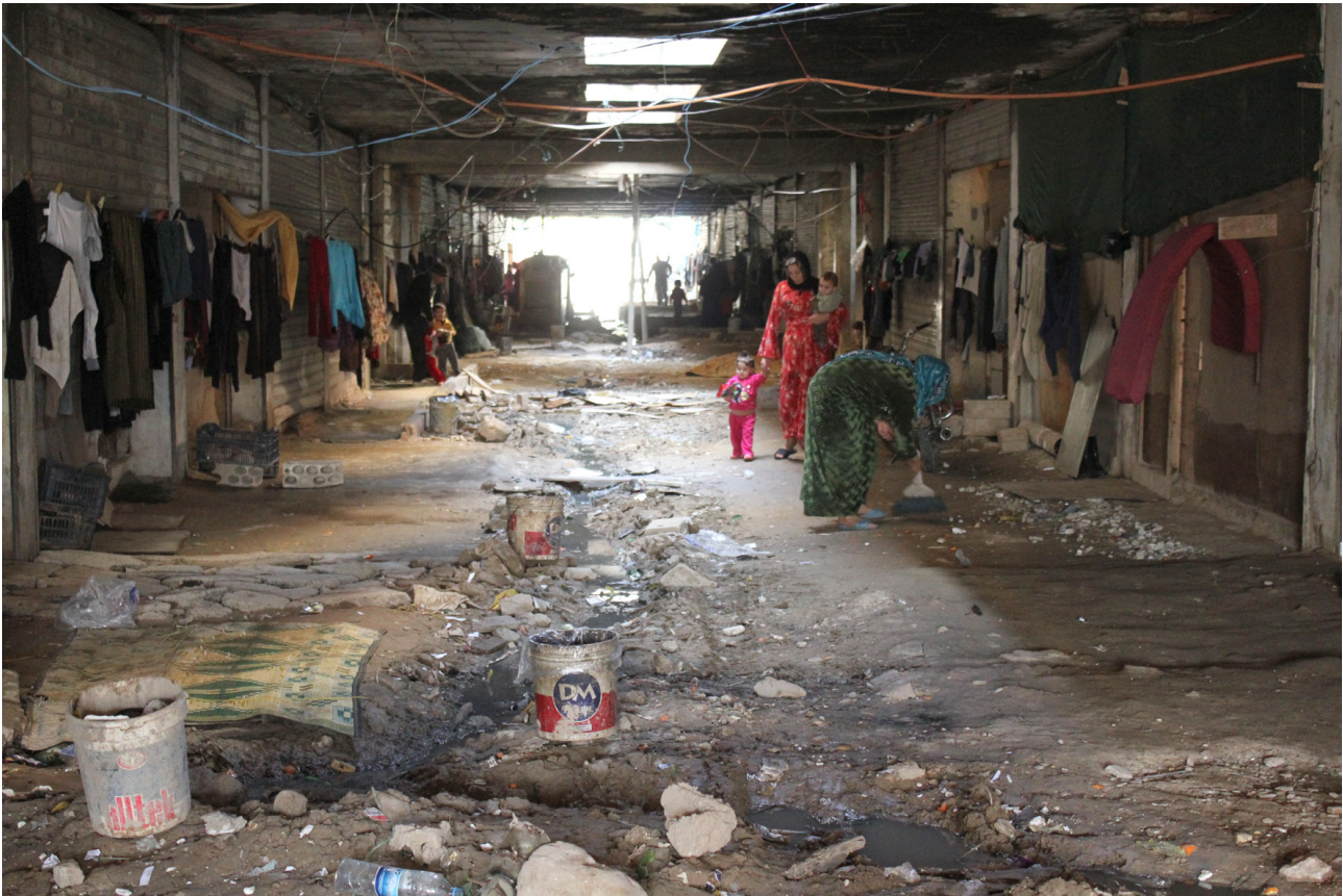
Figure 2. Picture taken in Aqbiye' collective shelter showing open sewage-channels running along the shelter units.
