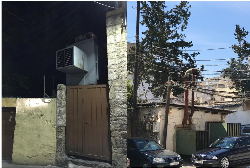
Figure 5.1. Generator Examples, Al-Mina
