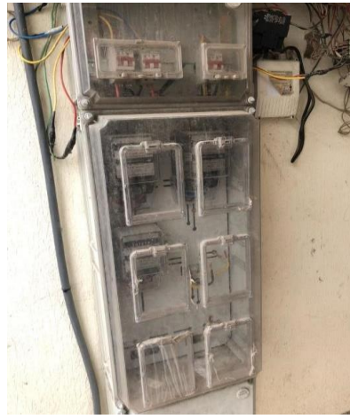
Fig. 13- 14: Old meter boxes VS. new meter boxes, 2018 Source: Author
