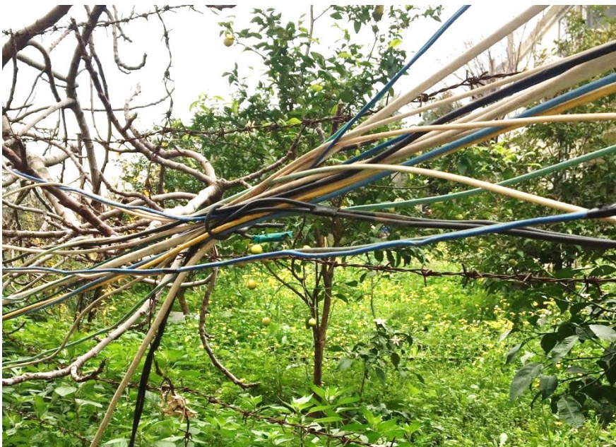
Fig. 26: Intertwined cables held together with a duct tape.
