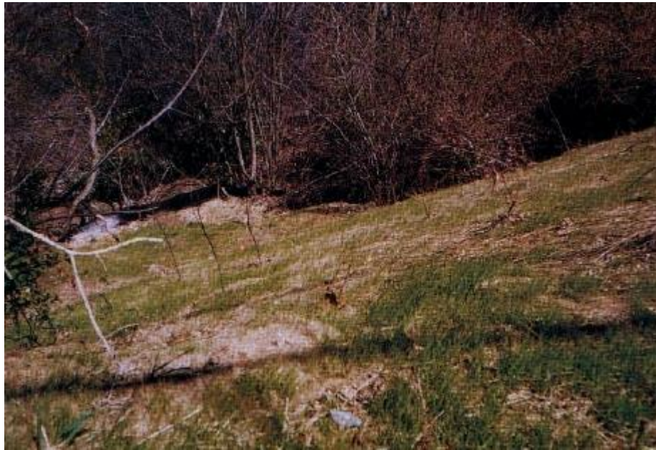
Figure 1.4 Repaired slope using Geofibers (from GEOFIBERS job report – Riverview drive slope reconstruction)
