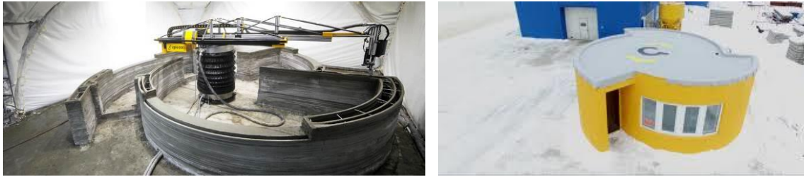
Figure 8. Apis Cor printed home. (1) In process of printing, (2) Apis Cor printed home covered with insulating material and paint.
