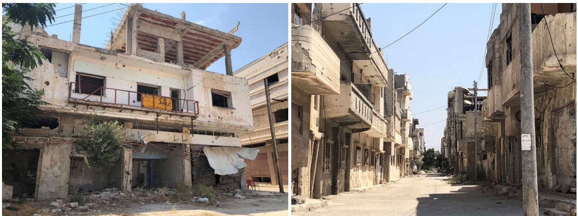
Figure 82: Low levels of damage ( Source: the author )
