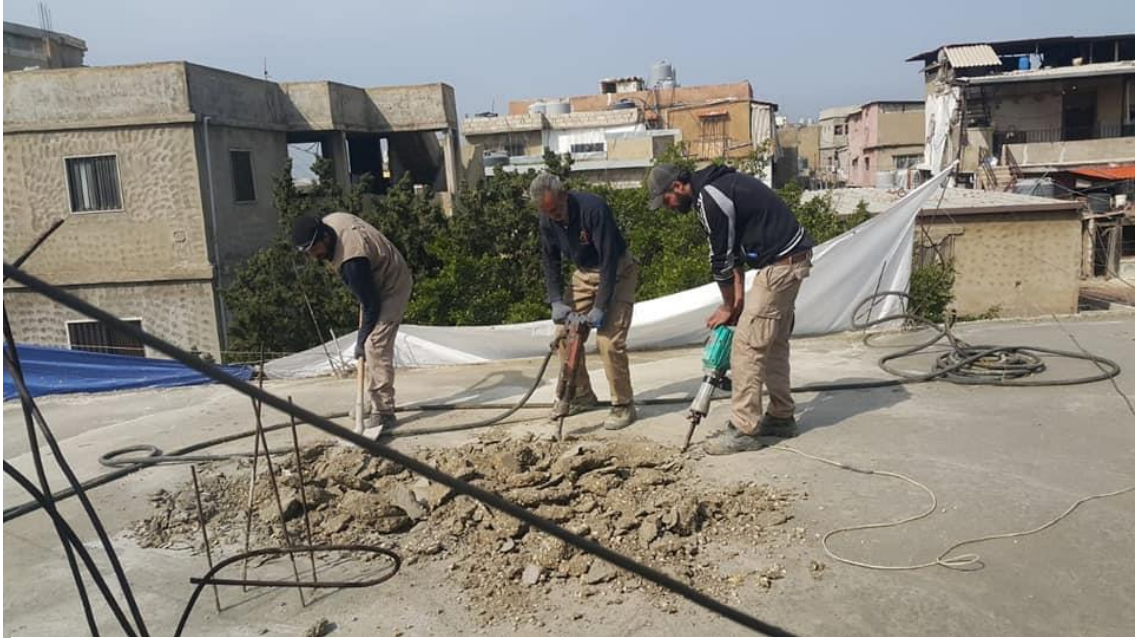
Figure 19. (2019). Removal of a building violation in Ouzai in Borj municipality. [Digital Image]. Source: UMD's Facebook page.
