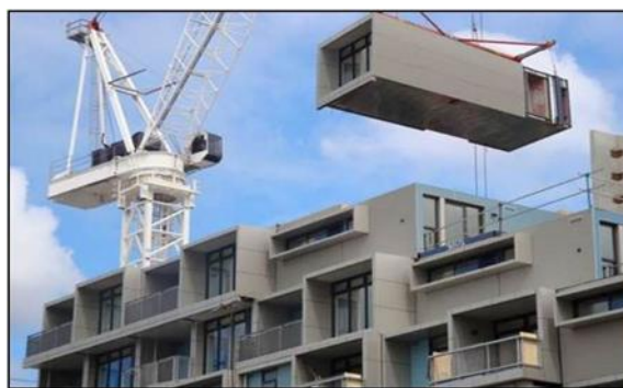
Figure 18 – Placing of volumetric units to complete block of flats (Hashemi et al., 2016)
