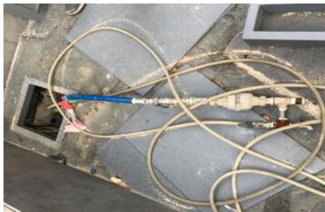
Old Water Gauge Connection JD 233, September 2017
