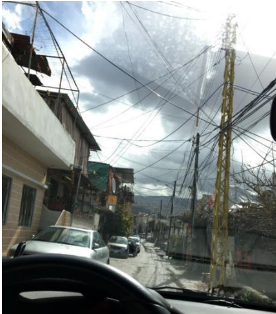
Figure 19: Web of Electrical wires inside the camp, 2017 (Source: Nadine Salhab)
