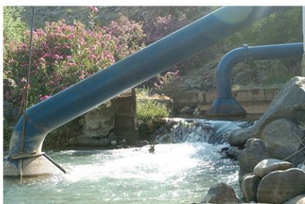
Wazzani Pumps project and sewage water plant implemented for Hasbaya village only 2002
