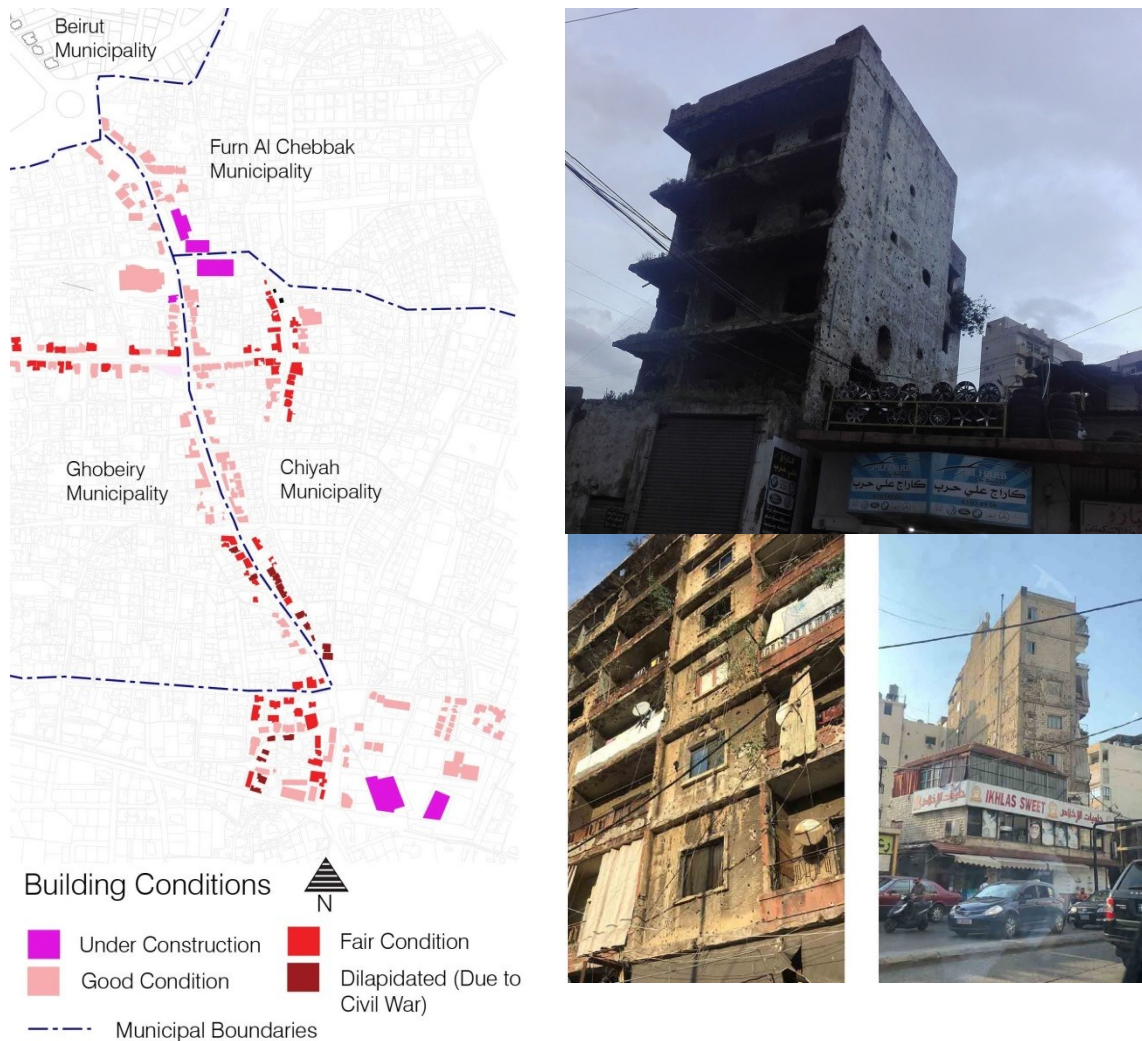
Figure 21: Building conditions along the edge zone of Old Saida Road (left), and images showing dilapidated buildings due to the civil war in the middle section of the edge zone. (Author, 2019)
