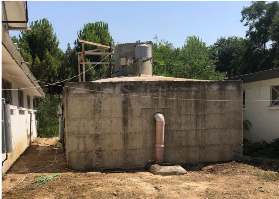
Figure 6: The anaerobic digester next to GPH
