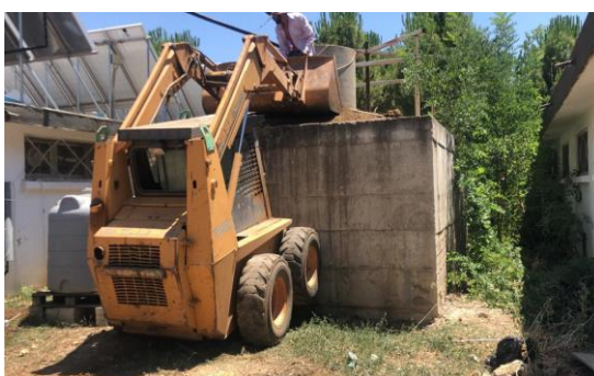
Figure 16: Loader emptying the manure in the digester
