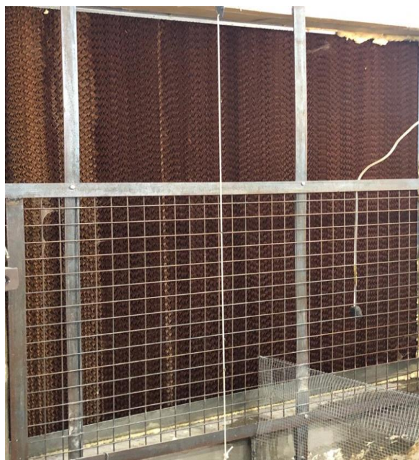
Figure 9: Cooling pad in CPH
