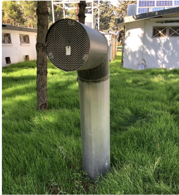
Figure 5: Geothermal heat exchanger
