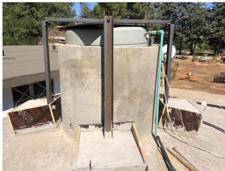
Figure 17: Steel cross base on the opening of the digester
