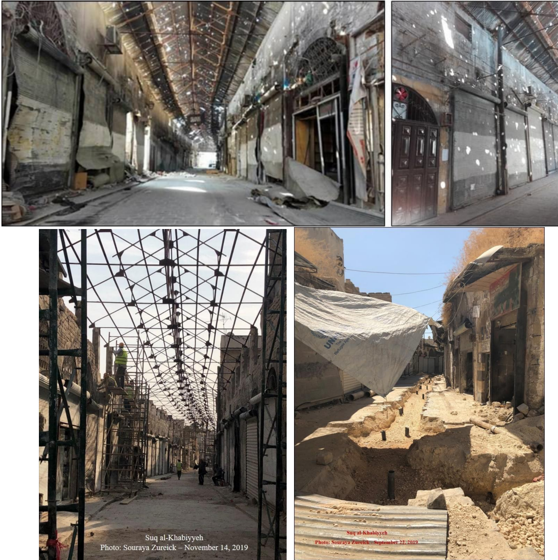
Figure 33- Photos of the Rehabilitation of Souq Al-Khabiyyeh Before and during the UNDP’s project (Top: the souq before the launch of the project, bottom right: the rehabilitation of the Souq’s infrastructure, bottom left: the rehabilitation of the shops’ facades). (Group of Students from the Faculty of Architecture in Aleppo (photographer), 2018; Souraya Zureick, 2019)
