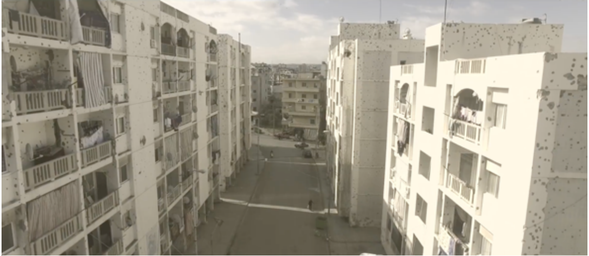
Figure 7 Image of one block of buildings showing the damaged façades – Source: footage from SHIFT NGO
