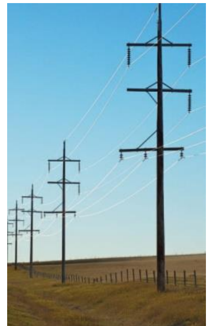
Figure 1.1 Timber utility poles.
