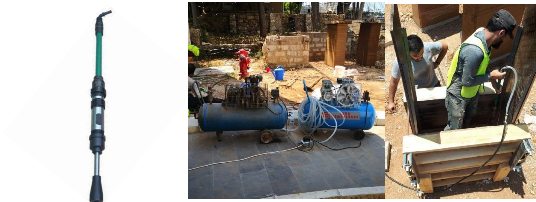
Figure 11 – Left: Pneumatic Tamper Used, Middle: Air Compressor Setup, Right: Ramming Using Pneumatic Tamper
