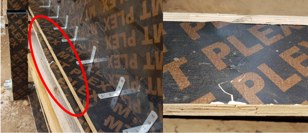
Figure 26 - Cracked Formwork and Deformation (shown in the red ellipse)
