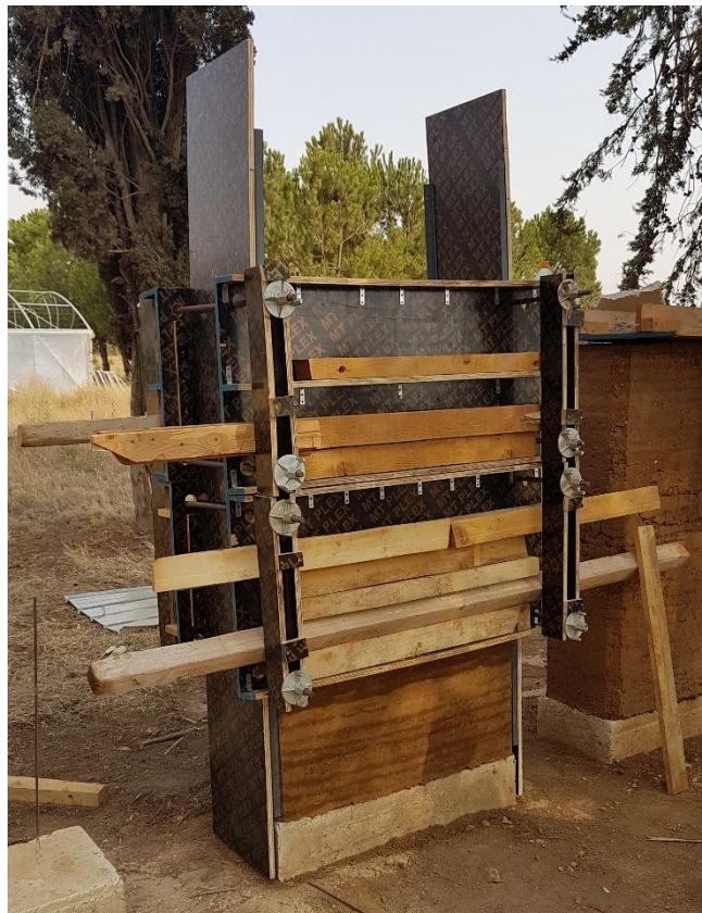
Figure 27 - Improvised Formwork Bracing System
