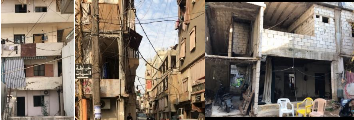
Figure 3. 16: Pictures showing the plastered, cladded, and incomplete buildings, photos taken by the author (2020).
