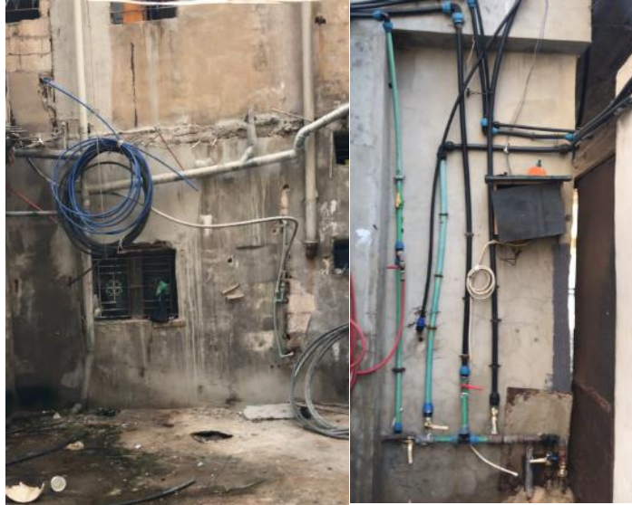
Figure 3. 18: Pictures showing the poor and exposed infrastructure, photos taken by the author (2020).
