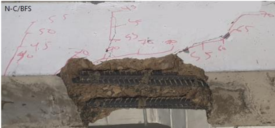
Figure 5.8 Failed splice region for beam N-C/BFS
