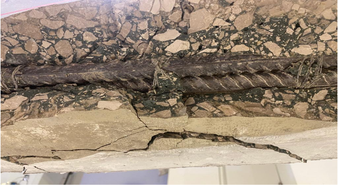
Figure 5.8 Failed splice region for beam N-C/BFS
