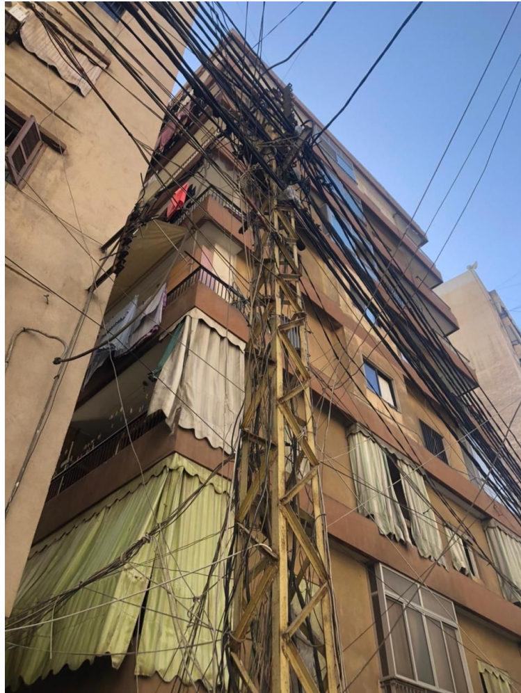
Figure 2. Messy visible wires
