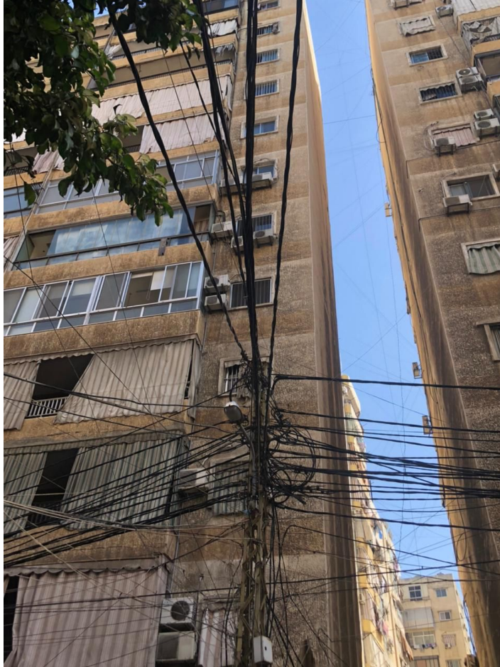
Figure 1. Messy visible wires (Photo by Danah El Kaouri)
