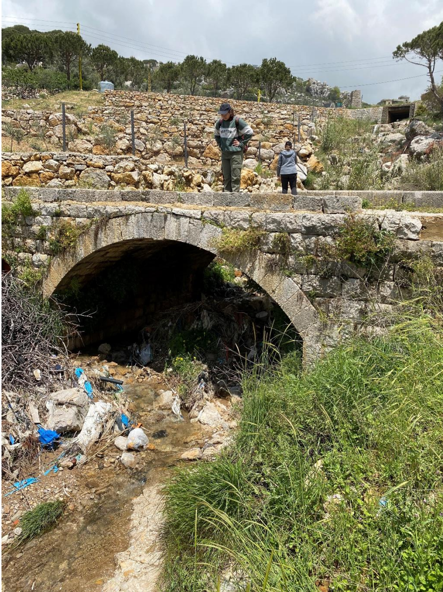
Figure 2.7. The northern bridge (MC02), currently used as part of the modern road network.
