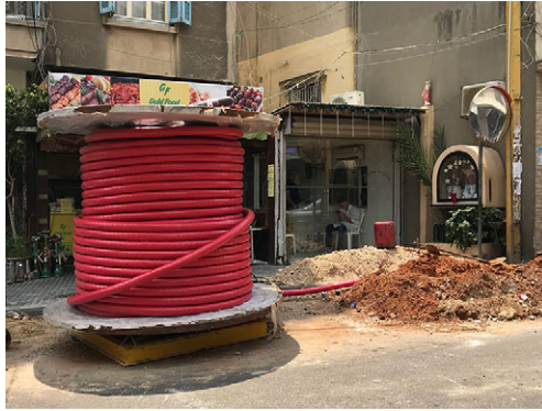
Figure 7 In the summer of 2018, Beirut residents experienced the arrival of fiber optic cables. Photograph by the author.
